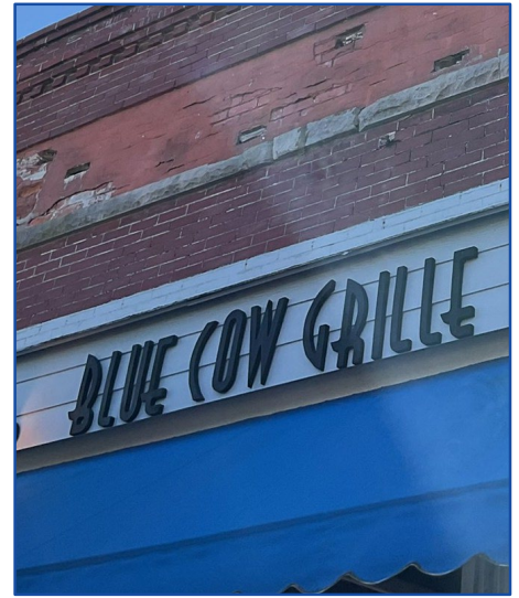
Fascia signs (above), window signs, and projecting signs (below) are appropriate for commercial buildings.
