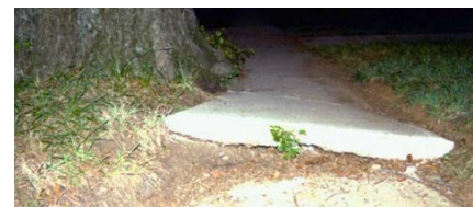
Figure 1: Extreme sidewalk lifting associated with tree roots
