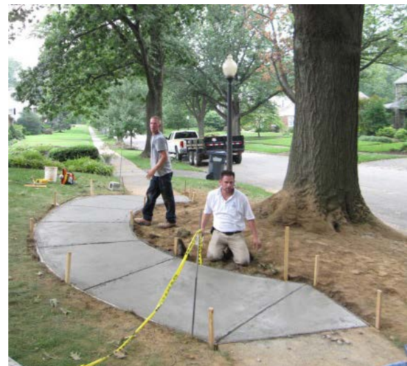
Figure 5: Sidewalk rerouted to increase the distance from the trunk and avoid root damage
