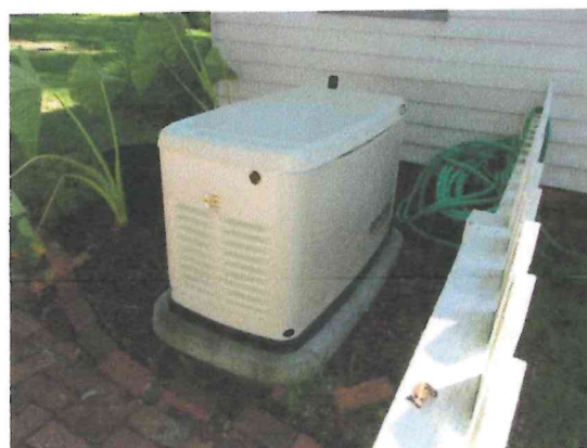
Whole House Generator
