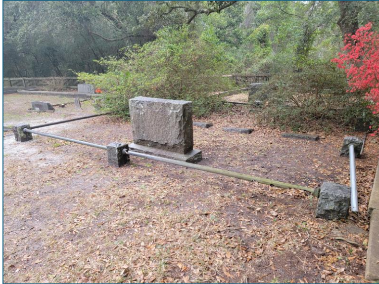
Decaying Galvanized Pipe Surrounding Gravesite
