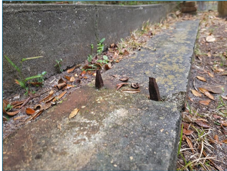
Decayed Fence Rails (Lower Coping Appears as a Step)
