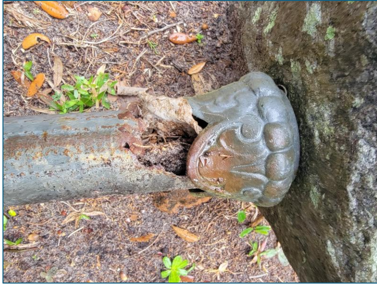
Corroding Pipe Ends
