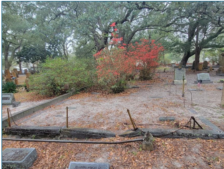
Broken Fence Posts & Broken Granite Coping
