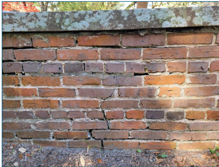
Brick Pointing Failing
