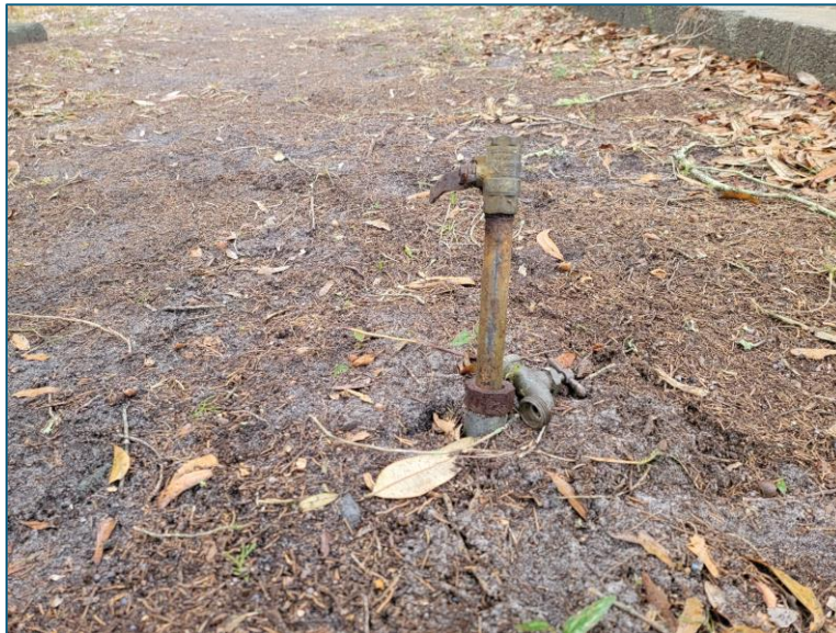
Broken Hose Bib in Pathway
