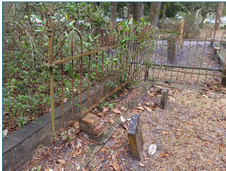
Fence Supported by Bricks
