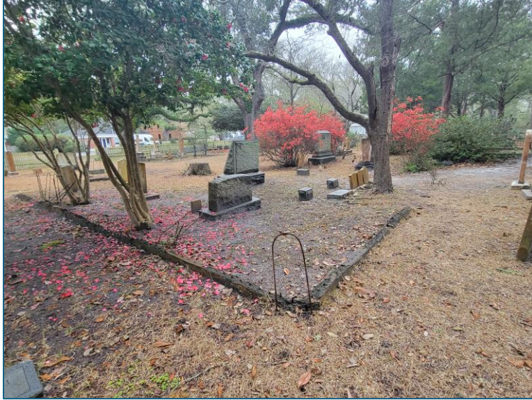
Decaying Coping and Fencing
