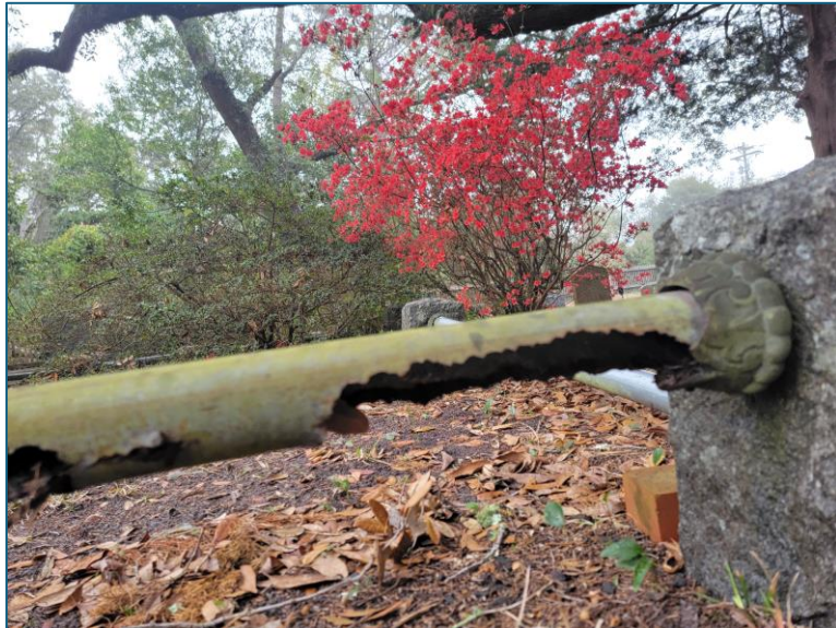
Corroded Galvanized Pipe
