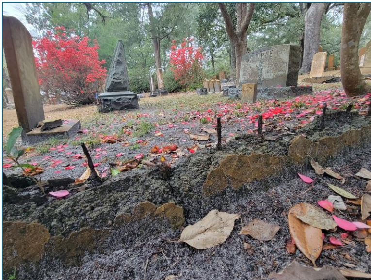
Decayed Fence Rails and Coping
