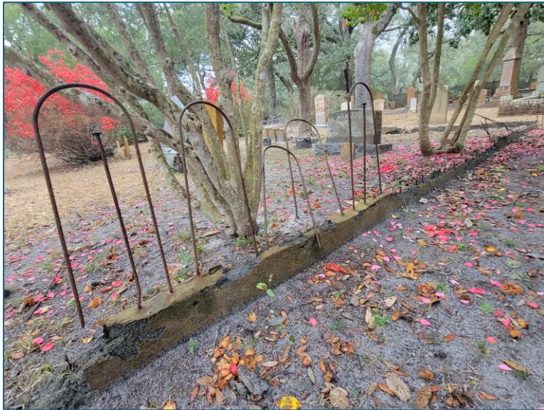
Remaining Fence Rails
