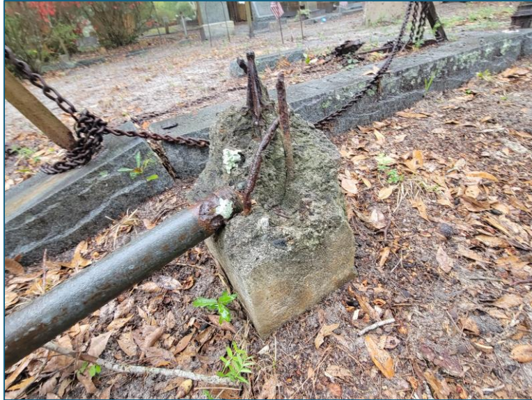
Broken Fence Posts with Rebar
