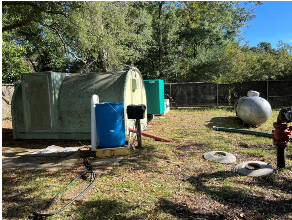
The City is currently designing pump improvements at the Leonard Street LS
